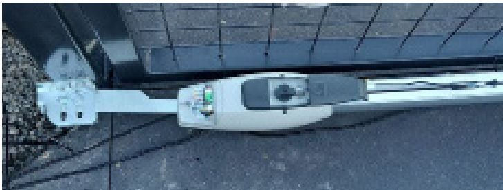
Incorrect setup showing the arm running parallel with the gate
