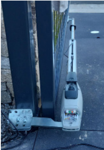
Incorrect setup showing the arm running parallel with the gate
