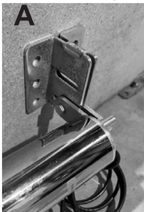
Image A & B incorrect setup
